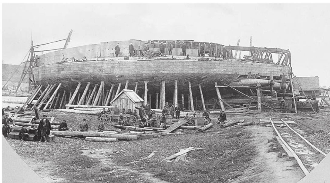
Another photograph of Popov under construction, this time from the port quarter. The framing for the after superstructure from the barbette to the stern is in place, as are the rudder and screws. Note the larger size and deeper placement of the inboard propeller. (Courtesy of Dmitry Lemachko)
