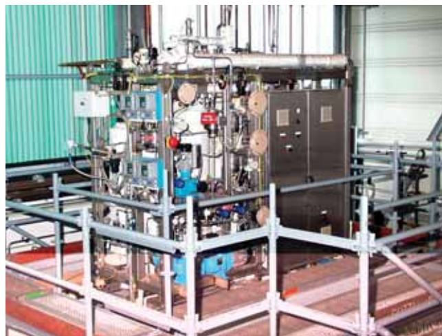
Functional Demonstrator of 240kW Methanol Reformer.
