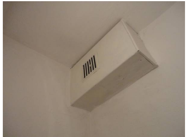
Picture#31: Replace ventilation system and put under new drop ceiling
