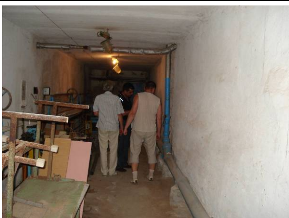
Picture#92: Sewer piping along the basement hallway to be repaired or replaced (1.4.2)
