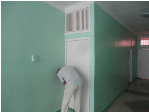
Picture#36: Replace door and louver for ventilation over the doors of the 6 bathrooms in West Wing
