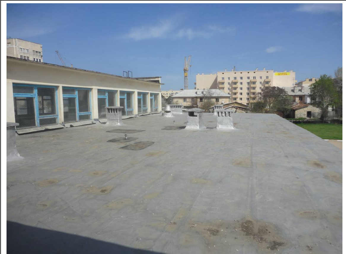
Picture#11: Roofing area to be repaired.
