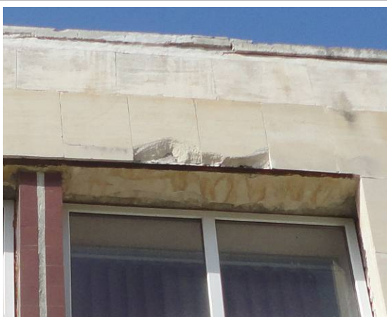
Picture#105: Typical broken natural stone tile. Top piece also to be repaired. Exposed metal to be repaired or covered. Top of window opening to be repaired like rest of plastered finished surfaces.
