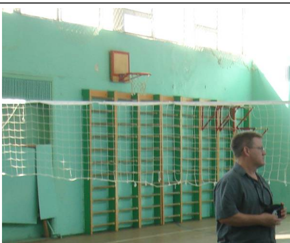
Picture#60: Existing wood racks and secondary basketball board to be replaced with new.
