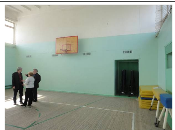
Picture#61: Gymnasium room with door to be replaced connecting with school entrance lobby
