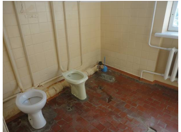
Picture#37: Typical condition of boys' toilets in West Wing
