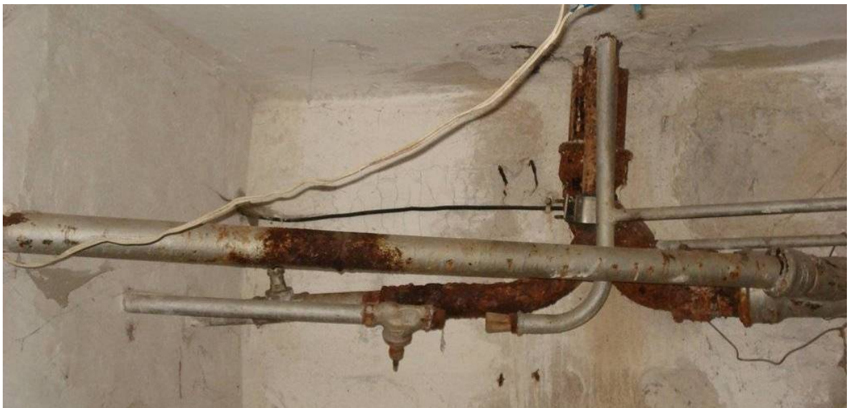
Picture#81: Typical condition of sewer lines in the basement. This corresponds to paragraph 1.4.1. All piping to be replaced with new PVC piping. Provide supports as recommended by the manufacturer.
