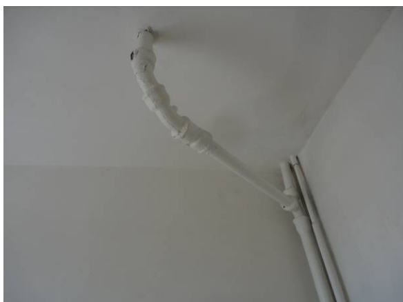
Picture#32: Typical drainage piping from floor above to be replaced with new PVC piping and covered under drop ceiling and new wall surfaces. No piping to be seen in bathrooms after renovation is complete.
