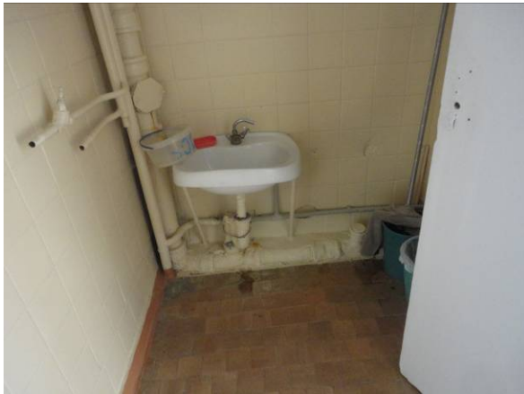
Picture#34: Typical sink in boy's bathroom of West Wing. Everything see in the pictures is to be replaced with new.
