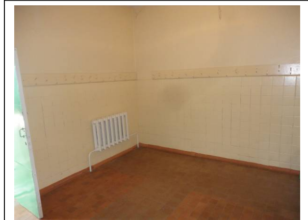
Picture#66: Interior of locker rooms. Replace radiators. Provide new ventilation to the exterior of the facility to avoid bad smell.
