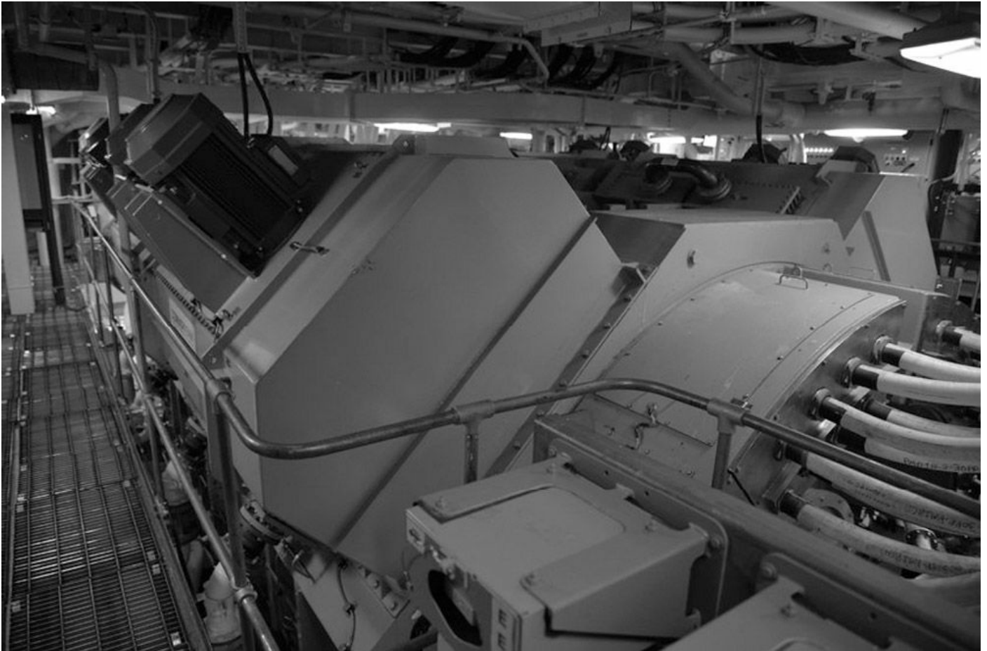
Two views of one of the two GE Power Conversion advanced electric motors that draw electrical energy from the Zumwalt class's integrated power system to turn the ship's fixed propeller shafts. The images show the heavy electrical cables connecting the huge motor to the ship's electrical grid and the direct connection between the motor and the propeller shaft: there is no need for a traditional gearbox. (Christopher P Cavas)
